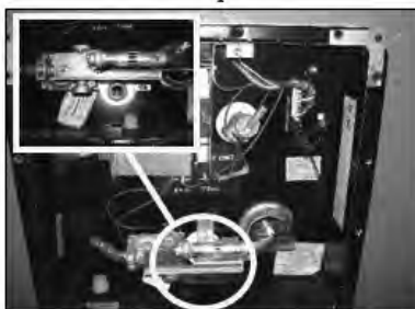
Fig 1: Water Heater Drain Plug
