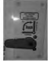
Water Heater Bypass
