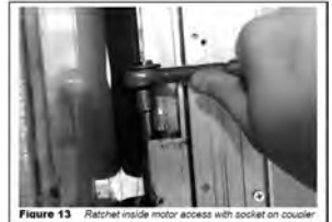
Figure 13 Ratchet inside motor access with socket on coupler
