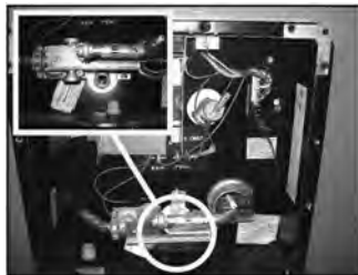
Water heater drain plug
