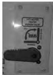
Water Heater Bypass
