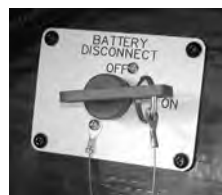
Battery Disconnect Switches
